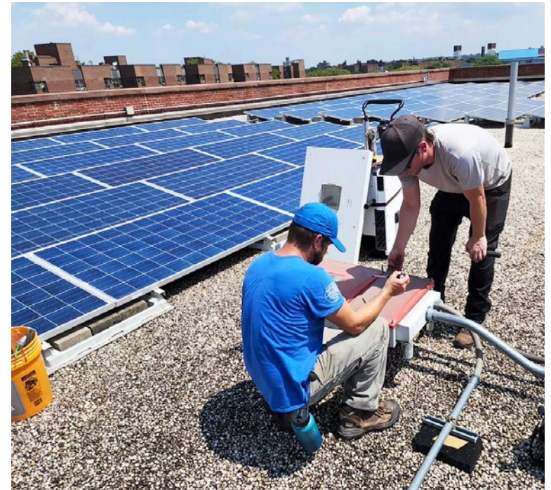
Two technicians work on the solar array at Franklin Delano Roosevelt High School (Brooklyn).
