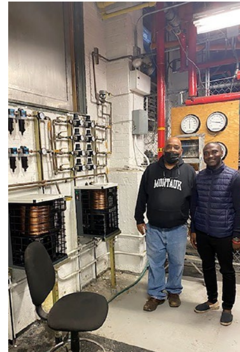
Office of Sustainability Energy Program Manager Desmond Ofori poses with Custodian Engineer Terry Harris of MS 246 Walt Whitman (Brooklyn), who received lighting upgrades and a Pneumatic Line Repair thanks to Demand Response funding.
